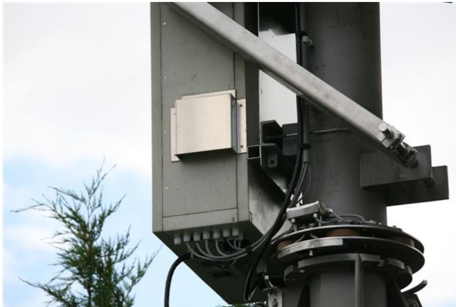
Figure 2: The bottom AZ bearing with the AZ limit switch and equipment box (note the air exhaust for one of the two PA bricks)
