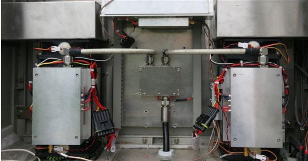
Figure 6: Two power amplifiers combined in the hybrid coupler (centre)
