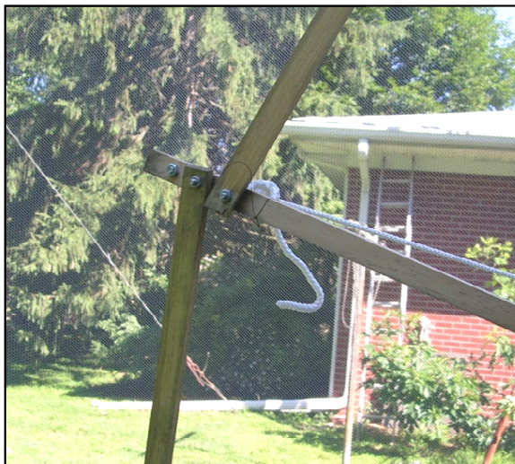
Figure 6: An outside rim is formed from 3.5-ft lengths of \frac{1}{2} " x \frac{1}{2} -inch modeling strips.
